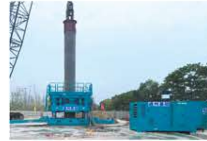
Nanjing Electric Power Company Continuous wall project of the underground pipe gallery
